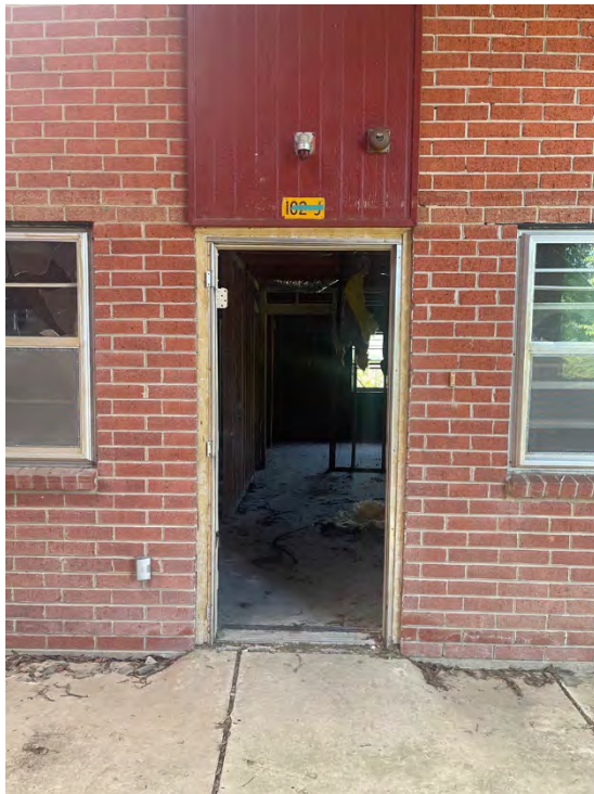
Photo 8. View of interior of damaged housing unit
