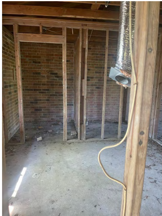
Photo 4. View of interior of damaged housing unit.
