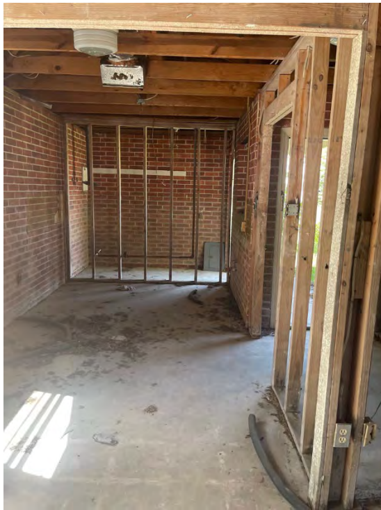
Photo 6. View of interior of damaged housing unit
