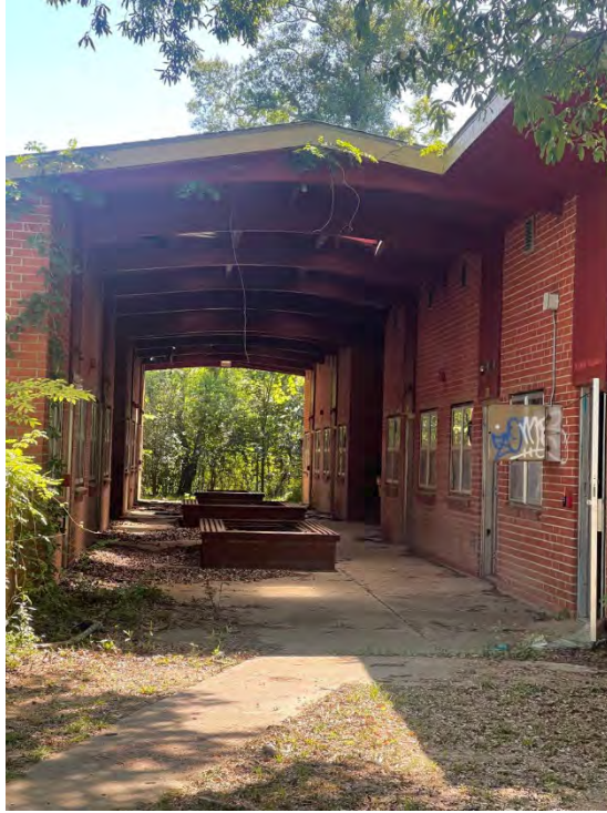
Photo 7. View of existing damaged courtyard at housing building # 102.
