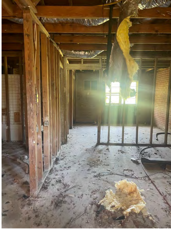
Photo 9. View of interior of damaged housing unit
