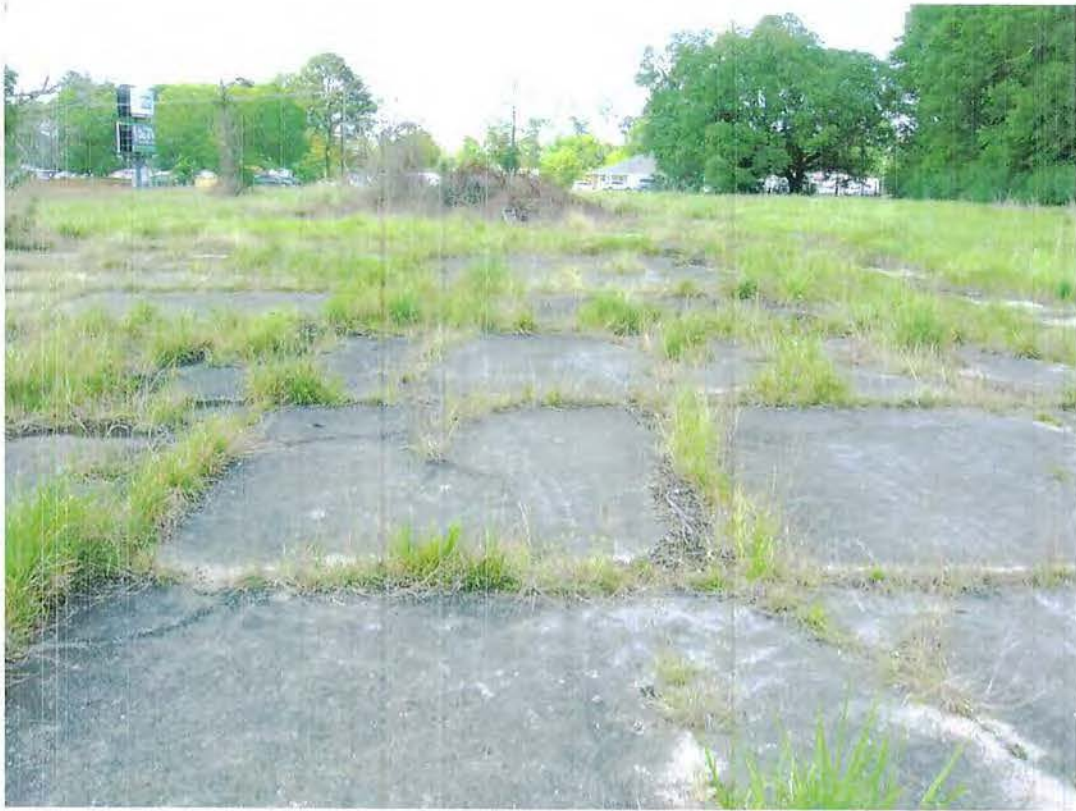
Remnant concrete slab found on-site.
