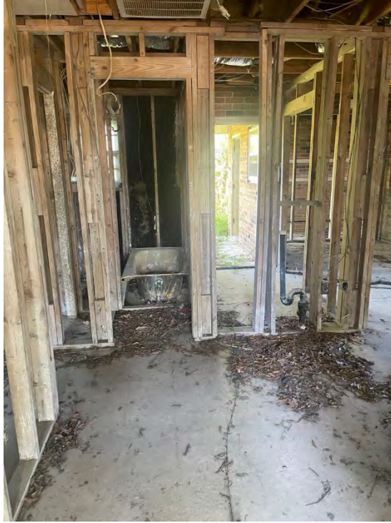
Photo 5. View of interior of damaged housing unit.
