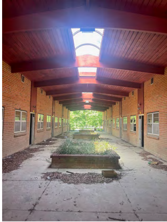
Photo 11. View of existing damaged courtyard at housing building # 102.
