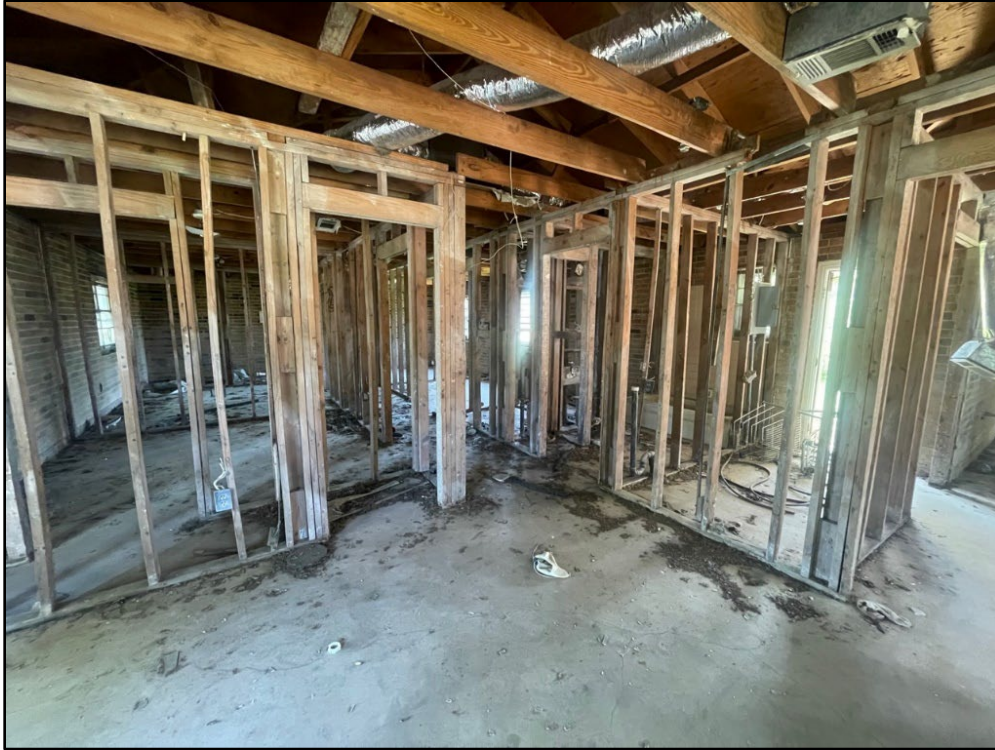
Figure 5 – Interior of damaged housing unit.
