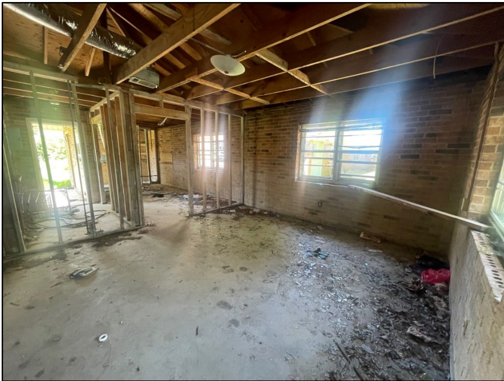
Figure 4 – Interior of damaged housing unit.
