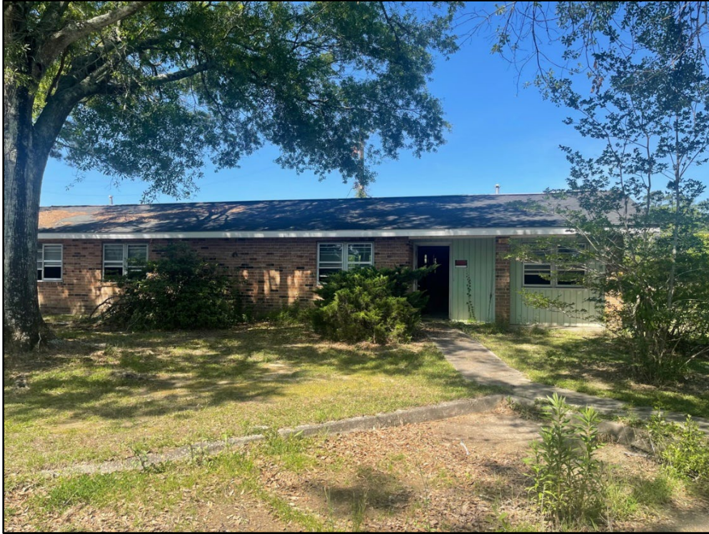
Figure 3 – Unoccupied/damaged housing building located at original facility location at 600 Eugene Street.
